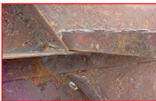
Rusted Surface before Rust Contact V Applied
