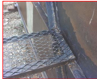
Rusted Surface before Rust Contact V Applied
