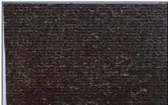
Rusted surface after application of Rust Contact V applied
